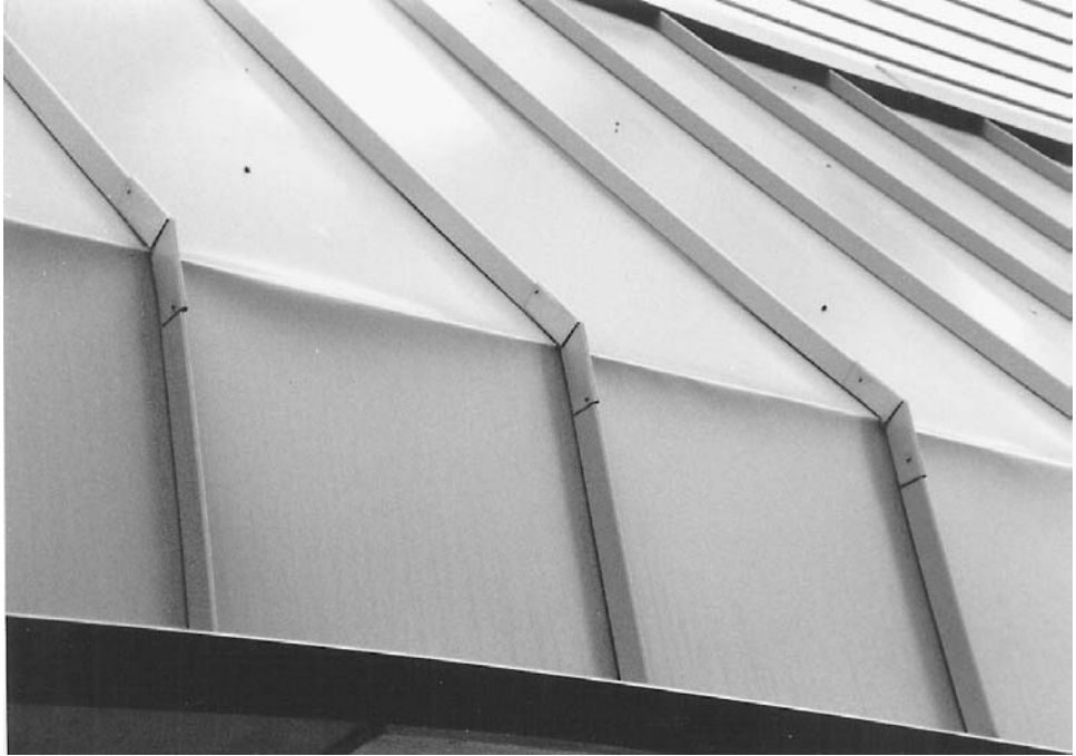
FIGURE 6.35 The line of roof-to-fascia transition occasionally comes out less than crisp.
